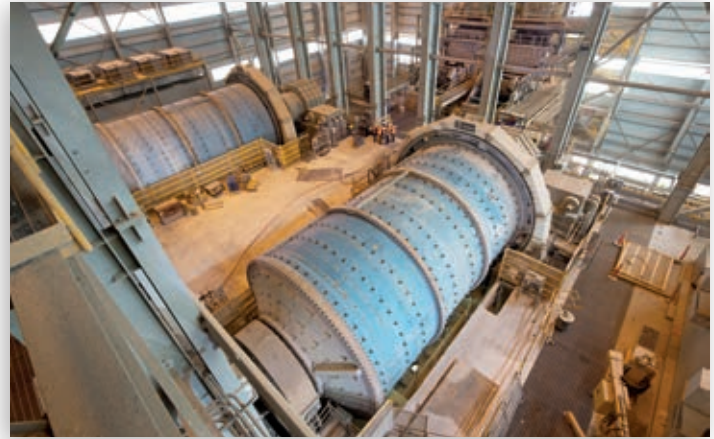
The Morenci mill expansion in Arizona commenced operations in May 2014. As part of the project, high efficiency ball mills and a hydraulic roll crusher were installed, allowing for the processing of higher volumes of ore with up to 25 percent more energy efficiency than other crushing circuits in the industry.
