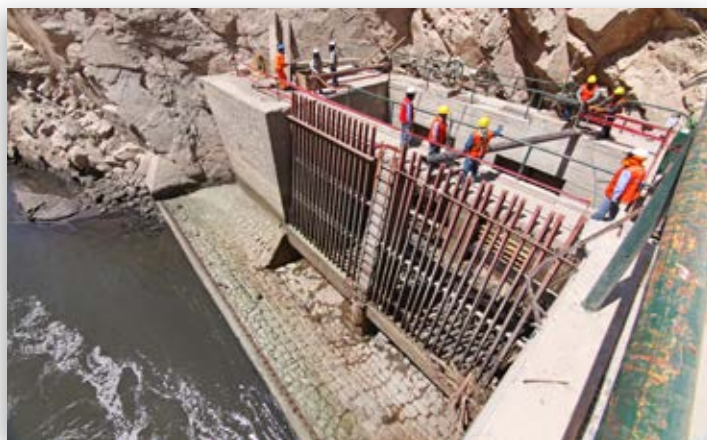
As part of Cerro Verde's work to improve water infrastructure within the Arequipa region, in 2014, it completed the reconstruction of floodgates on the Rio Chili. The new floodgates replaced antiquated infrastructure and help maintain the integrity of regional agricultural irrigation systems during severe precipitation events.
