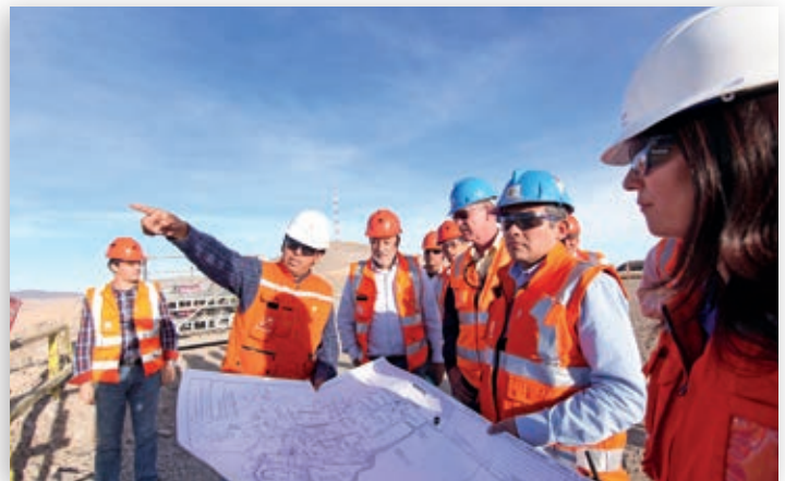
Former Minister of Energy and Mines of Peru, Eleodoro Mayorga (third from the left), and Cerro Verde management observe the construction of a wastewater treatment plant that will enhance water quality in the Arequipa region. The plant will supplement current water supplies to support the expansion of concentrator facilities to 360,000 metric tons of ore per day.
