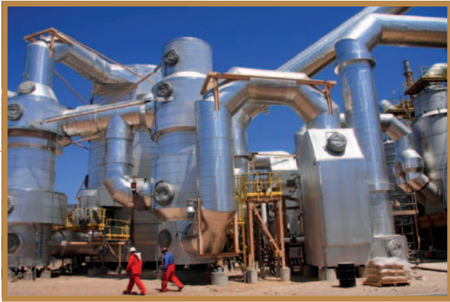
Photo: During 2011, we completed construction of a sulphur burner at Safford. The plant is providing a more cost-effective source of sulphuric acid used in copper leaching operations and results in lower transportation costs. Not only does the plant produce sulphuric acid, but the heat created in the process is used to produce high-pressure steam that drives a turbine to generate 15 megawatts of electricity. The electricity is being used by the plant and processing facilities, including the tankhouse, and will save the Company approximately $5.7 million per year in power costs.
