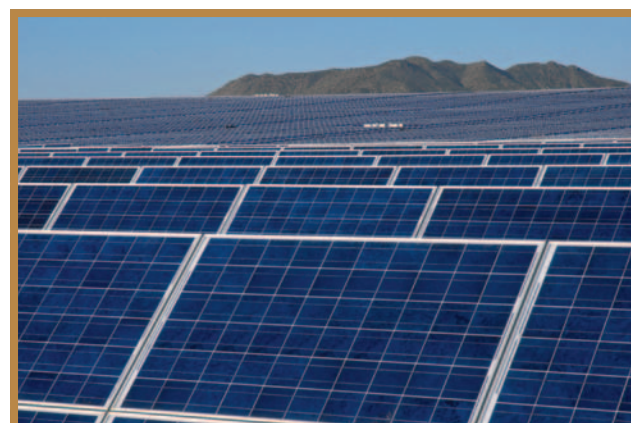
Photo: A 15.5-megawatt solar facility was commissioned on Company land in Bagdad, Arizona. Our Bagdad operation purchases the power generated at the facility, which accounts for 5 percent of the operation’s electricity needs and is projected to save the Company more than $700,000 annually. The facility is scheduled to operate for up to 25 years.
