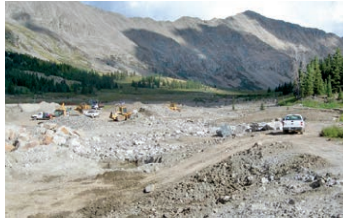
Channel excavation in the Storke Yard at Climax in 2007. The Storke Yard previously served the Climax mine for underground mine support.
