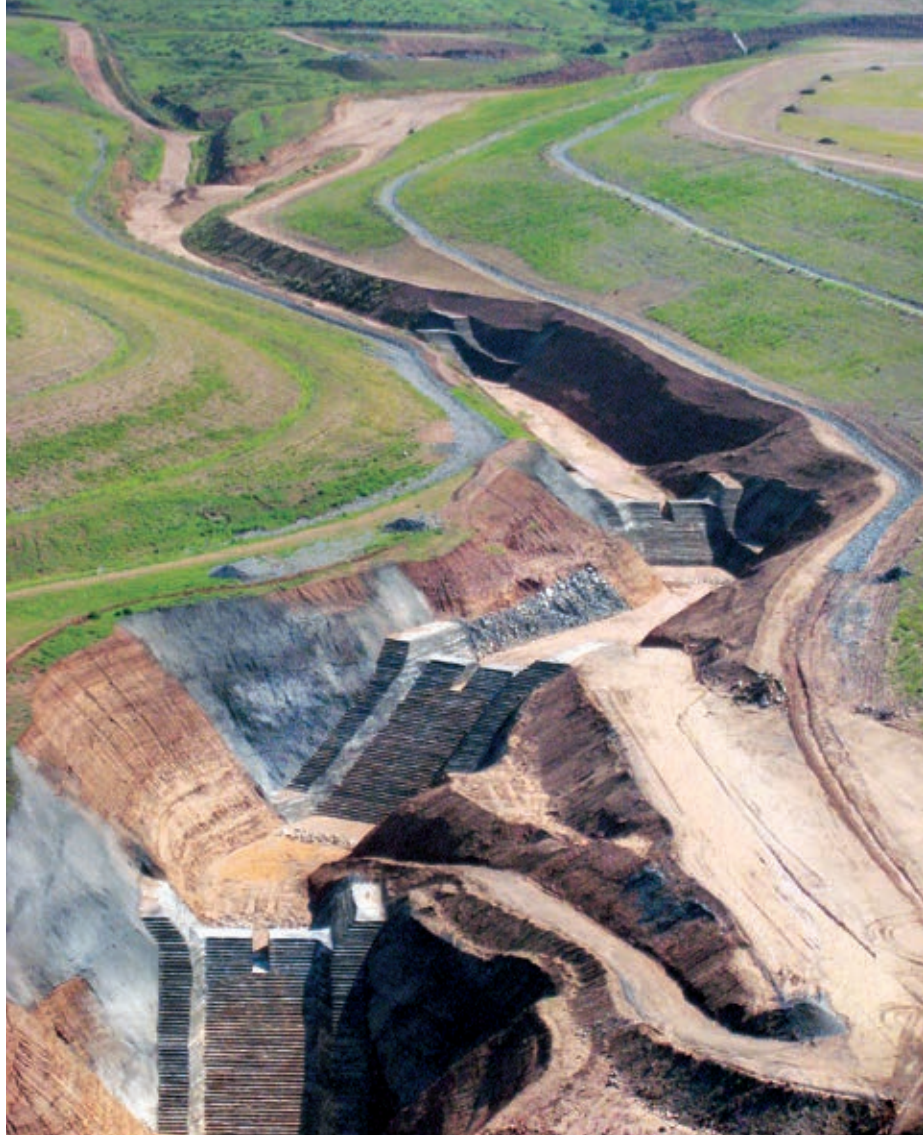
Erosion resistant cover materials in use at Tyrone. Stormwater channel armoring includes riprap, concrete block, grade controls, self-armoring materials and roller-compacted concrete.
