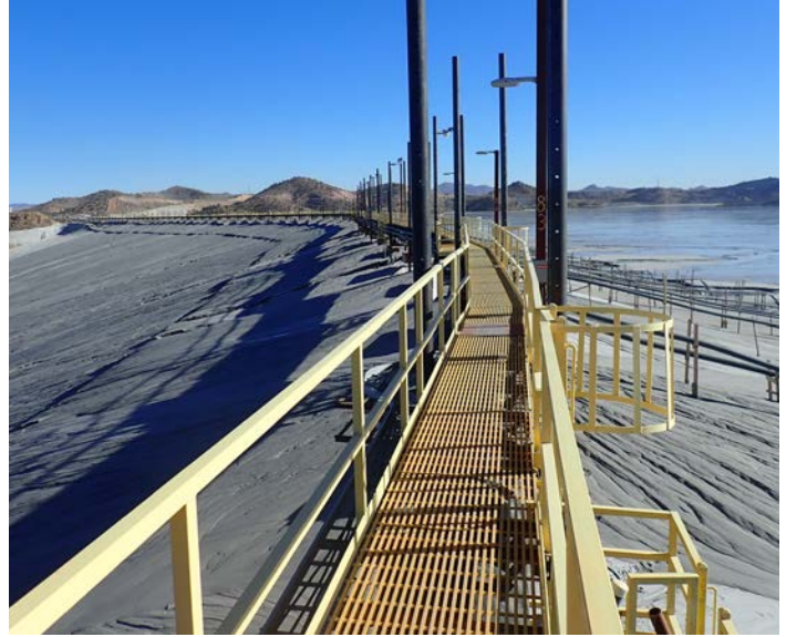
Above is the tailing distribution pipeline platform and jacking header along the centerline of Bagdad’s Upper Mammoth TSF. The platform supports 85 on-dam cyclones used to separate the material into coarse and finer fractions, where the coarse fraction is used to build a free draining embankment for the tailings storage facility.
