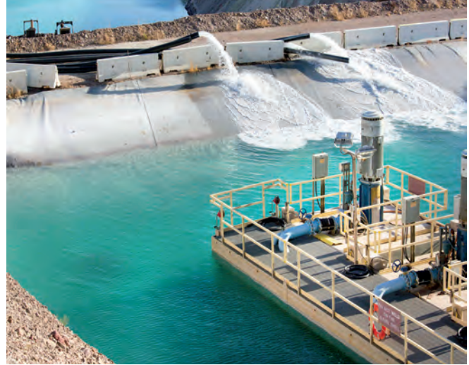
Barge pumps at Morenci transfer water from the tailings impoundment for recycling. The majority of our recycled water originates from reclaimed water captured at tailings facilities and leach pads.
