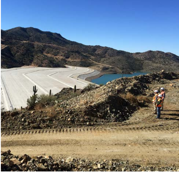
Members of the Tailings Stewardship Team (TST) inspect the Bagdad tailings dam as part of an annual audit. The TST is a multi-disciplinary group of internal and external experts that evaluate the design, operation and maintenance of tailings storage facilities. The company operates 18 active and 52 inactive or closed tailings dams.
